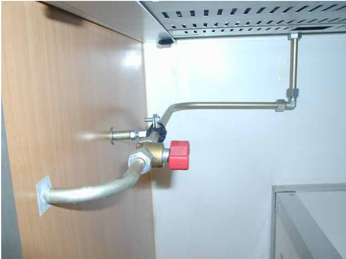
Example of good pipe work secured and grommeted at entry points
