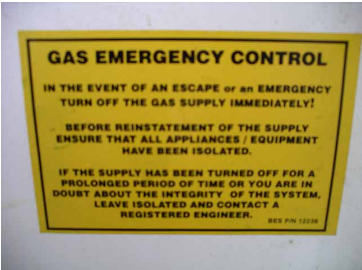
Example of a safety/warning notice (in the event of an emergency)
