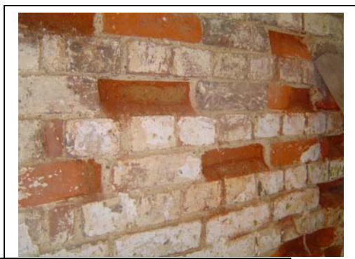
The use of a modern water resistant paint has resulted in the damage to this brickwork
