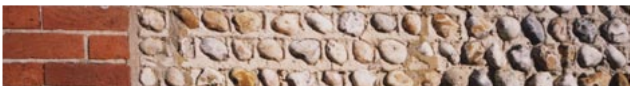
Whole flint cobbles and red brick are typical of the conservation area
